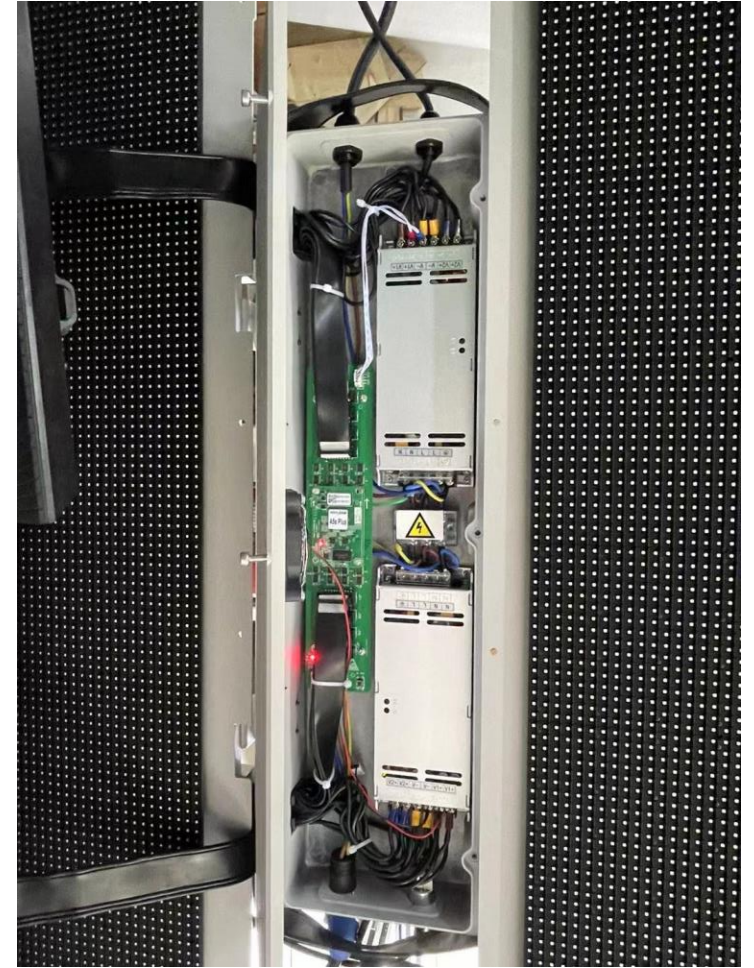
Inside of Power Box
